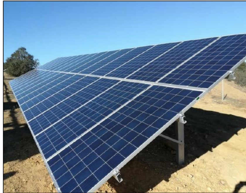
Typical solar PV Panels
