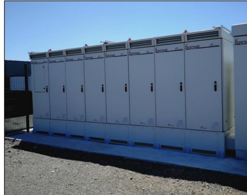
Typical centralised inverter
